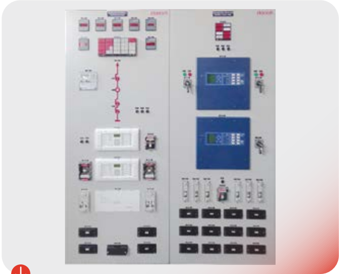
Control Relay Panels
