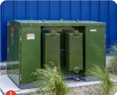
↓ Pad Mounted Transformers
