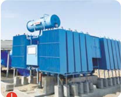
↓ Inverter Duty Transformers
